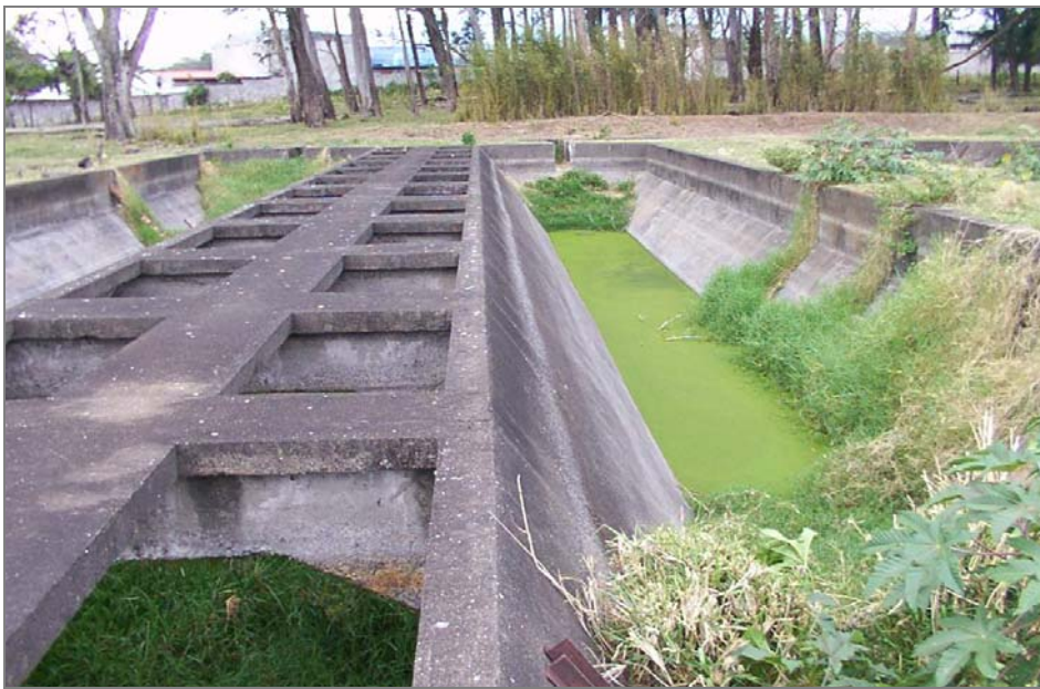
Tanque Imhoff (Biodigestor)
